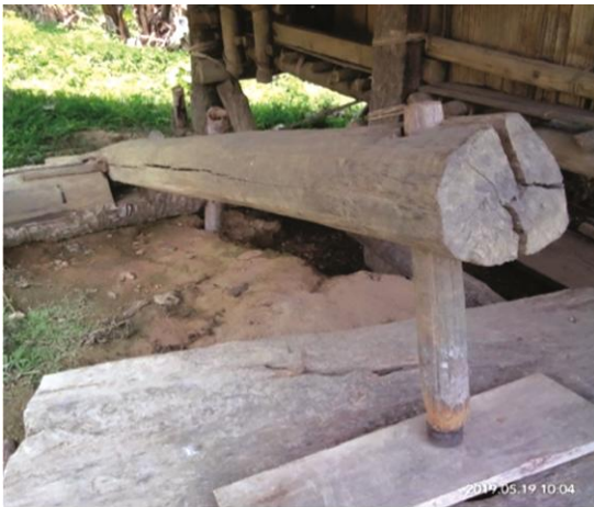
Fig. 8 —A mortar hole covered with wooden plank to protect from pollution and a prominent crack of the husking lever due to direct sunray
