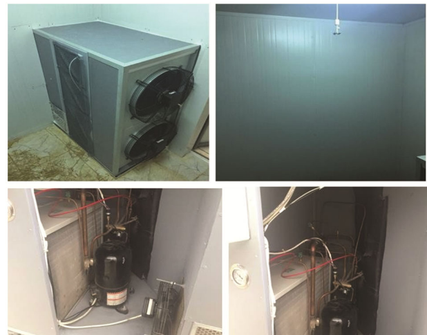
Fig. 1 — Unit room and air conditioning device
